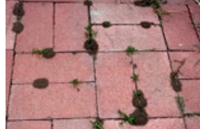
Pavement ant mounds in pavement seams
